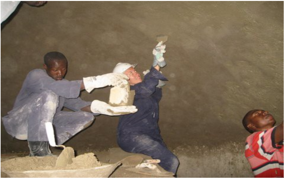
Illustrasjon 5: The tank must be waterproof at the bottom and gas proof at the top. This requires skilled masons to perform proper work.
